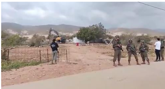
Still from demolition video. Click here to see video (source: Roni65043634 on X)
